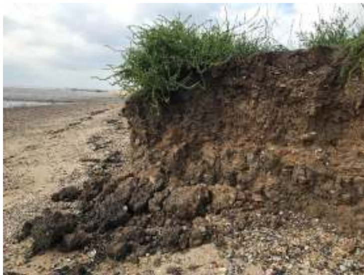
Figure 8. Detail of collapse of eastern tip of the fort ramparts. Image facing south
